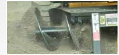
Coclea idraulica per lo spostamento del materiale Hydraulic auger for moving the material during excavation activities
